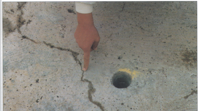
FIGURE 16 - CRACKING IN CONCRETE
